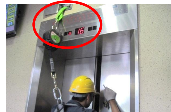
Permanent anchorage to access lift pit
